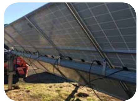
As you can see in the image, the module leads are significantly longer than needed for this application. Careful routing of the excess wires is paramount in this situation due to the lack of attachment points.
