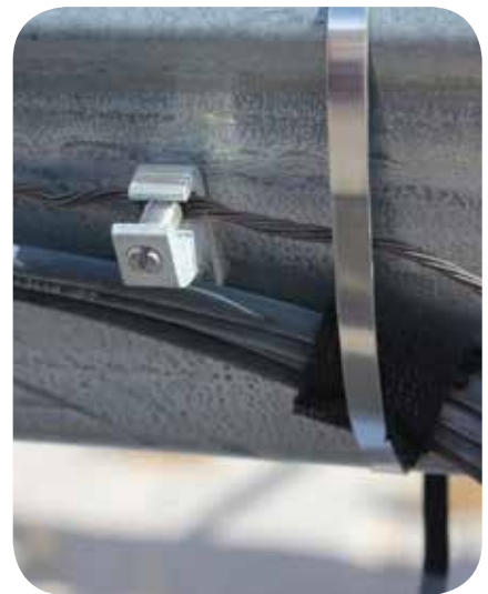
In the image above, effort was made to protect the cable jacket from potential abrasion from a metal cable tie. The fear is that this small piece of insulation may erode or slip and leave the cable jacket exposed to the metal tie at an unfortunate angle.
