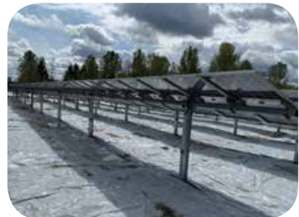
This project in Oregon utilizes a white ground covering to both increase UV radiation to the back of the modules as well to help mitigate growth of weeds and other ground coverings.
