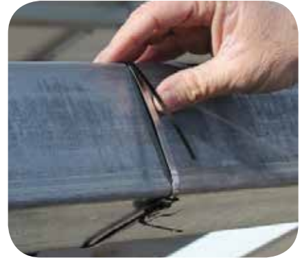
Vinyl coating separating from stainless steel cable tie.
