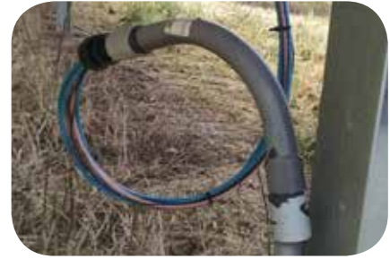
This conduit was damaged when the tracker went to the far east position every morning. The conduit also penetrated the module backing and cracked the glass.
