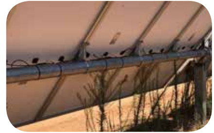
Longer ties are required for dressing wires along the torque tube. Care needs to be taken to make sure that proper materials are specified due to the high temperatures the torque tube can experience. Seen in this photo is the HellermannTyton 22 in. "Torque Tube" Solar Tie, part number 111-01196
